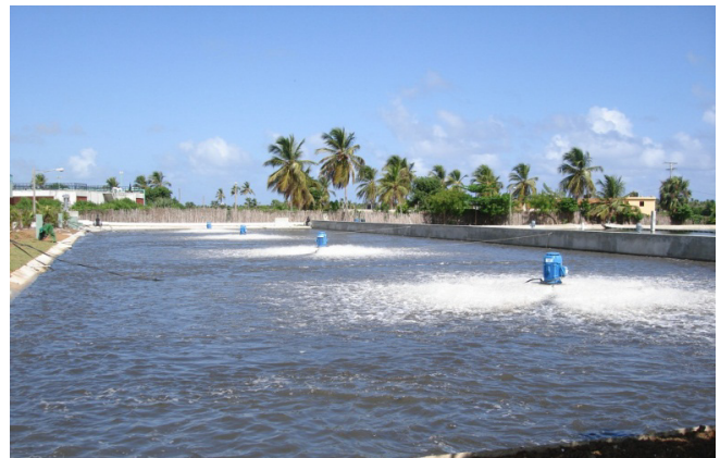
Typical TYPHOON installation in a lagoon
