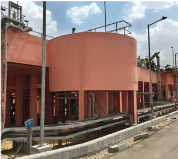
HUBER Vortex Grit Chamber VORMAX installation with HUBER Grit Washer RoSF4.
