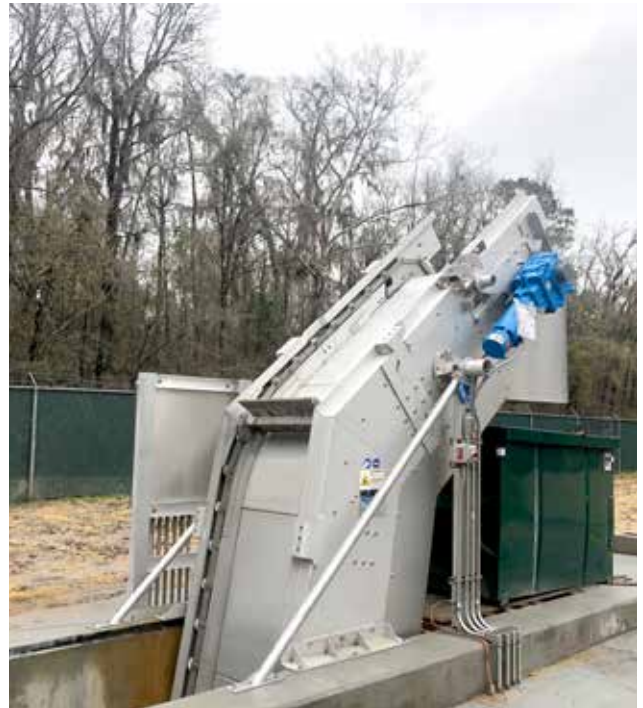
Screen installation in the inlet of a pumping station with discharge directly into a container.
