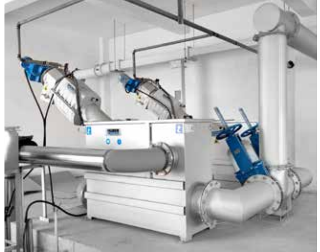
Tank installation of a HUBER Micro Strainer ROTAMAT® Ro9.
