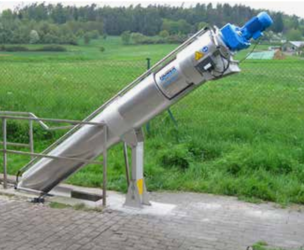
Outdoor installation of a HUBER Micro Strainer ROTAMAT® Ro9.
