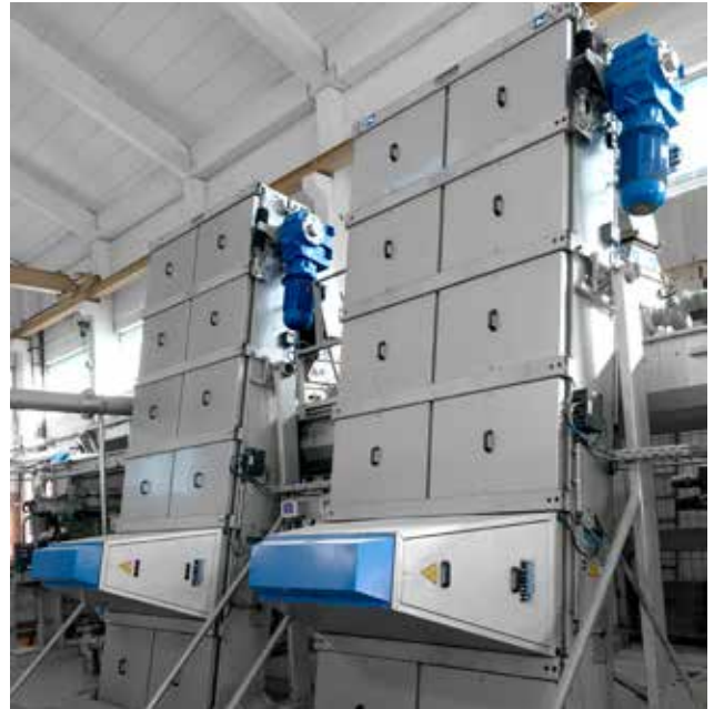
Two HUBER Multi-Rake Bar Screen RakeMax® units equipped with the HUBER Detection System Safety Vision. By detecting critical screenings, Safety Vision prevents damage to the screen and downstream machinery.
